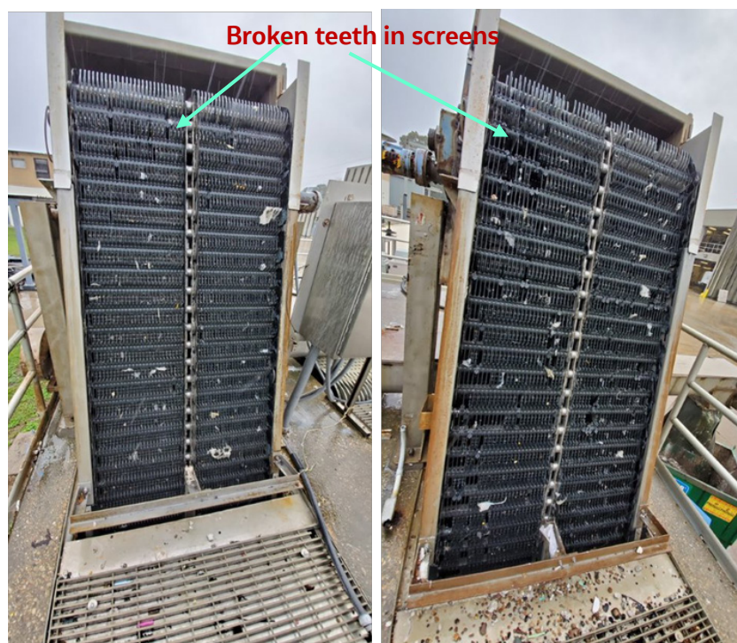
Figure 3-1. West Biloxi WWTF Headworks Screens
