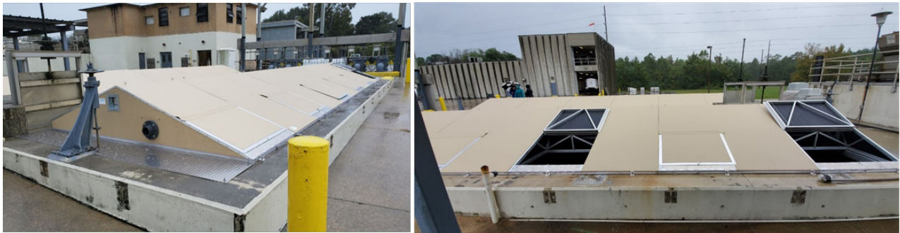
Figure 3-2. Aerated grit removal system at the West Biloxi WWTF out of service since 2004
